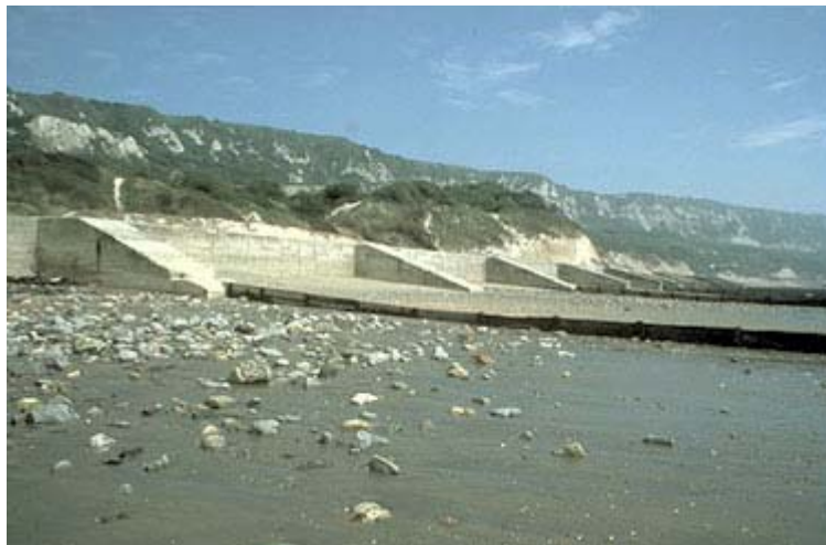
Figure 2.10 The foreshore at Folkestone Warren showing the toe protection and the undercliffe behind
