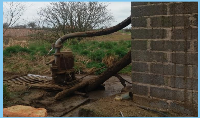
Slurry pump to supply the separator. Water is added to the slurry at this point to aid the separation process (approximately 36m 3 /month of added water).
